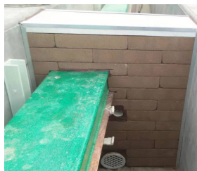
电缆沟阻火墙 2 (FS-Z 阻火模块系统)
